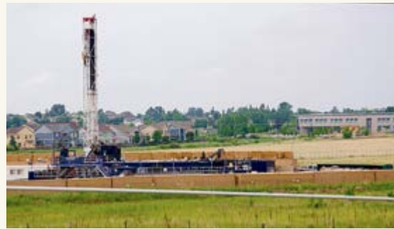
Thousands of spills of toxic chemicals or produced water have been documented in Colorado. Here, a frack site neighbors a subdivision in Erie, Colo. TOPHER DONAHUE
