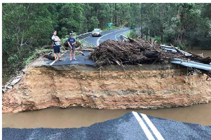
Figure 95: Damaged road in Queensland as a result of ex-Cyclone Debbie in 2017 136
