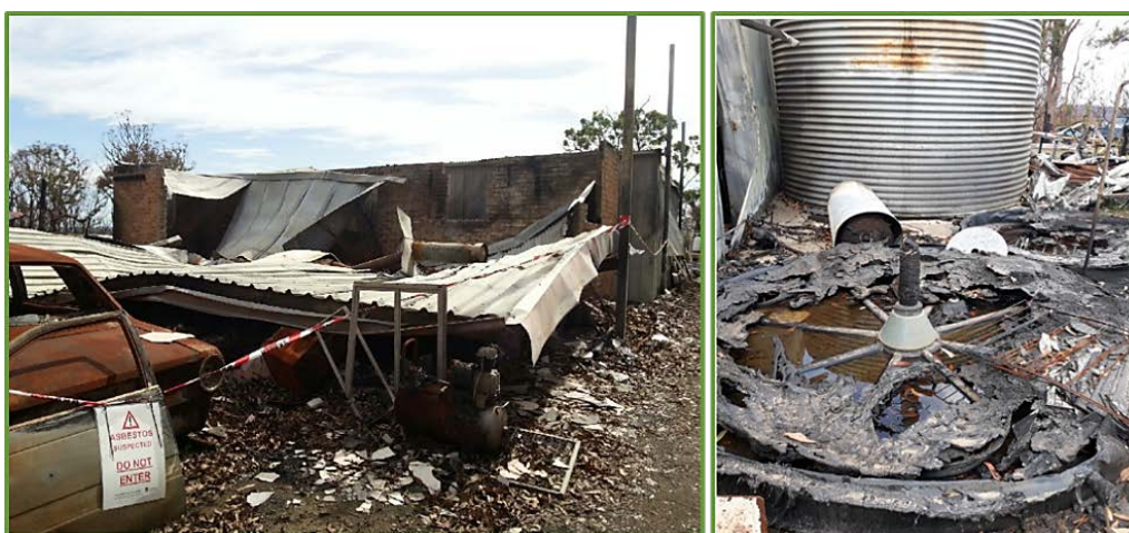
Figure 83: The presence of asbestos can add significant complications to clean-up efforts 58
