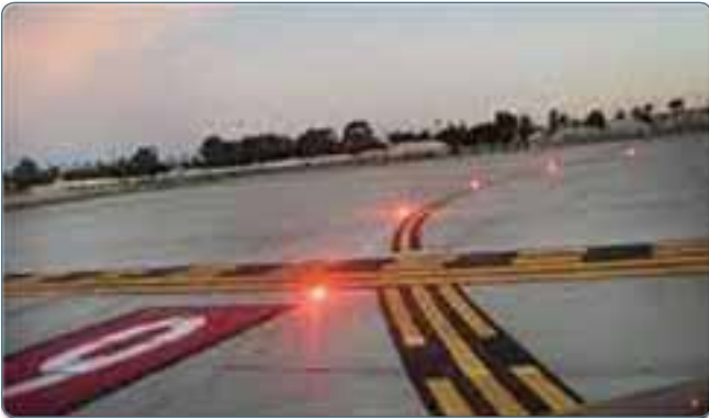
Figure 14-35. Runway Entrance Lights (REL).
