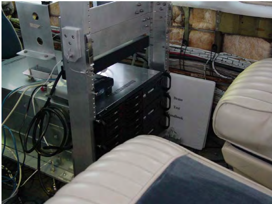
Figure D-5. The ATDSS I Data Recorders and Detection and Tracking Processors in the Aero Commander Cockpit
