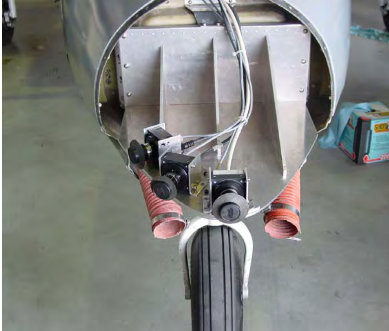
Figure D-4. The ATDSS I Sensor Installation in the Aero Commander
