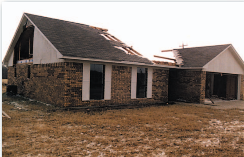
This house was damaged in a tornado near Whitehouse, Texas, on November 15, 1987. The damage would be rated EF1 on the Enhanced Fujita Scale.
